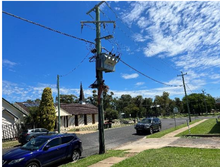
Picture 1 – Pole mounted transformer located in Reservoir Street
